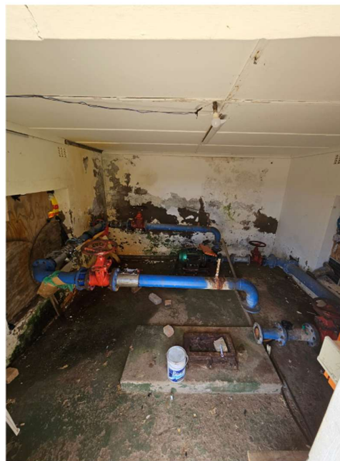
Figure 1: Kenton - Pumphouse for Elevated Tanks
