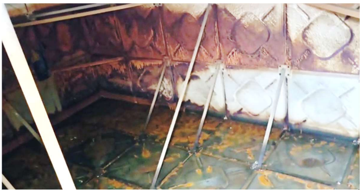
Figure 3: Poor Condition of inside of Elevated Tank
